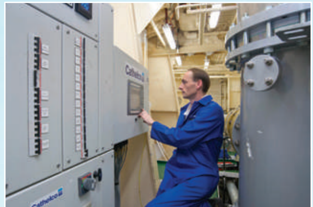
Paneles de control
